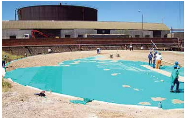
Tank Farm - Depósito Fuel Oil. Montevideo - Uruguay
