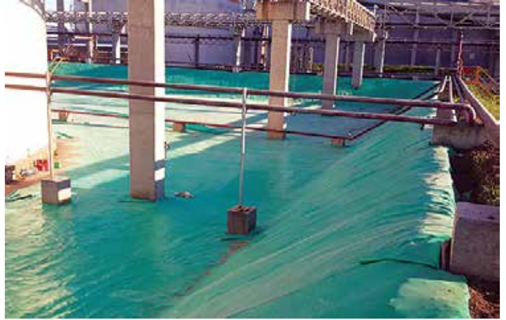
Tank Farm Noble Grain - Timbúes, Santa Fe
